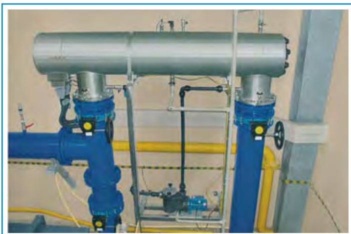
WTP, Kalish, Poland, 8 400 m 3 /day
