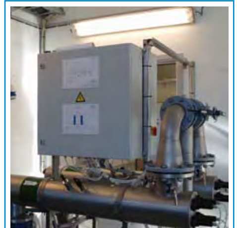
WTP, Rolvsvåg, Norway, 1 000 m 3 /day
