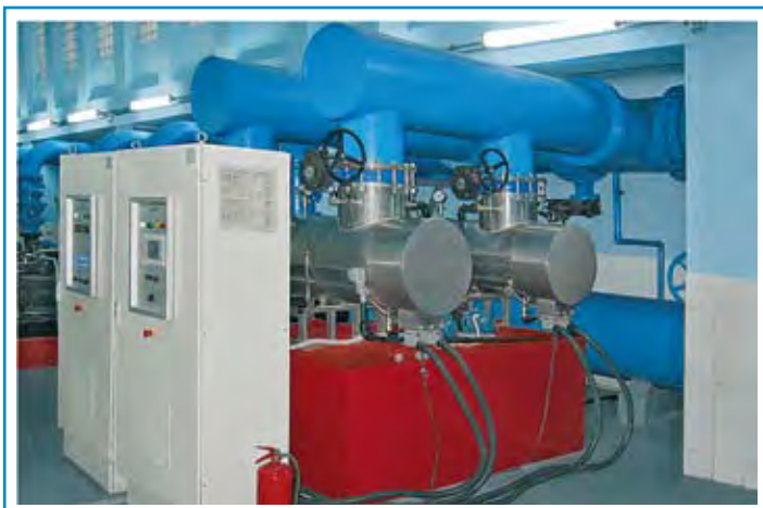
WTP, Calarasi, Romania, 36 000 m 3 /day
