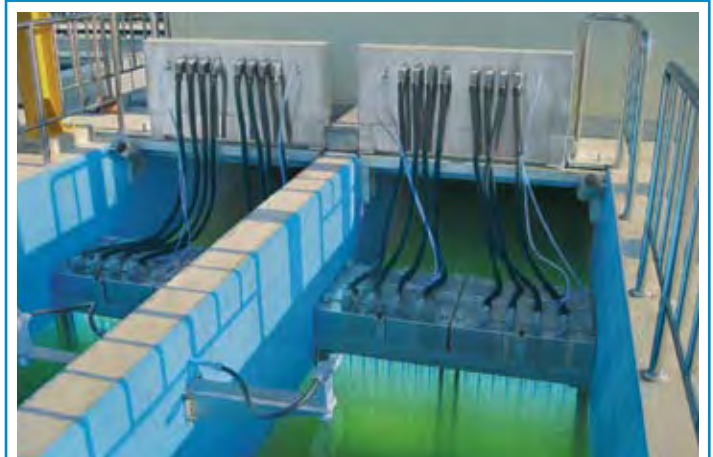
WWTP, Jeonju, South Korea, 120 000 m 3 /day
