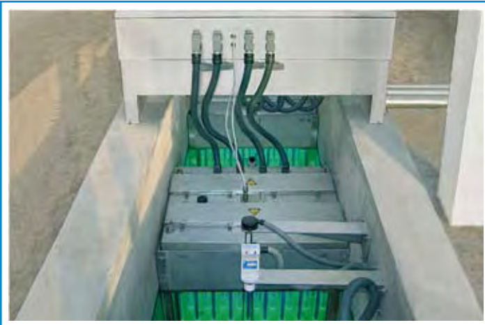
WWTP, Gadong, Brunei, 58 200 m 3 /day
