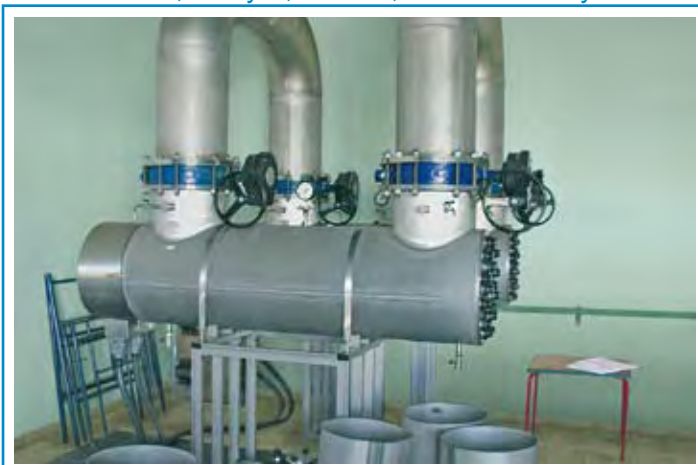
WTP, Granada, Spain, 24 000 m 3 /day
