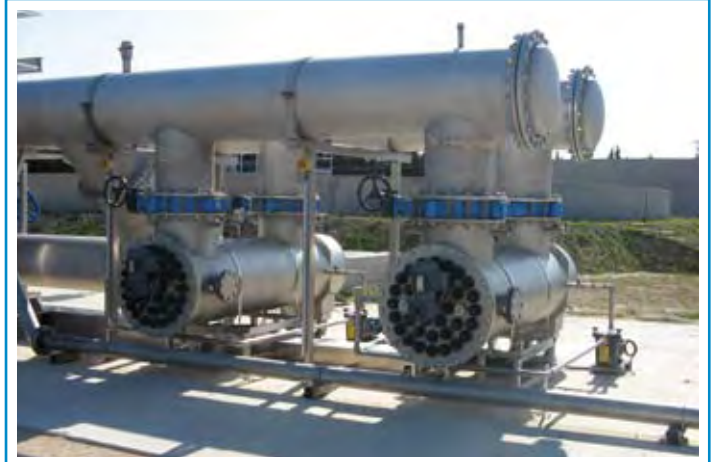
WWTP, Orange, France, 22 500 m 3 /day
