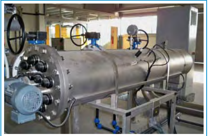
WWTP, Guadalix, Spain, 2 050 m 3 /day
