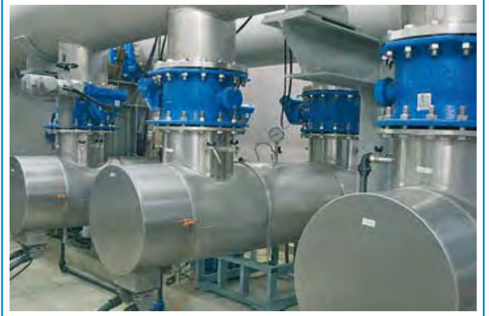
WTP Budapest, Erd station, Hungary, 48 000 m 3 /day
