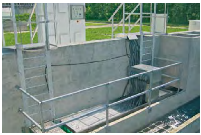
WWTP, region of Balaton, Hungary, 18 200 m 3 /day
