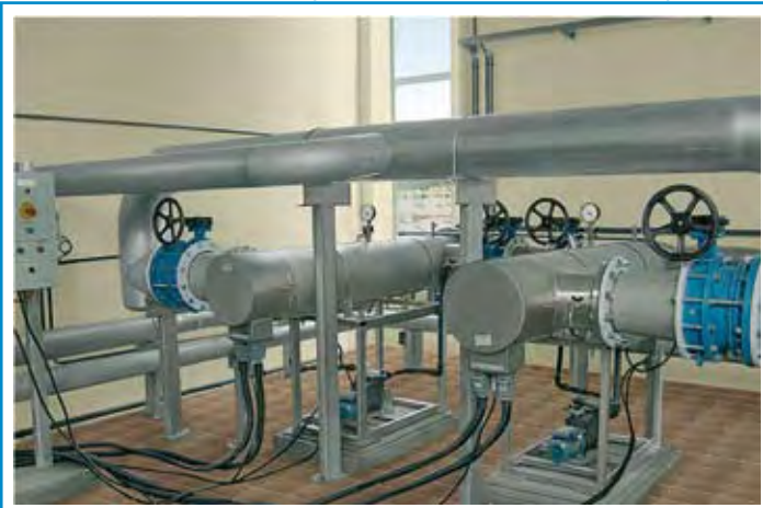
WWTP, El Endrinal, Spain, 24 500 m 3 /day
