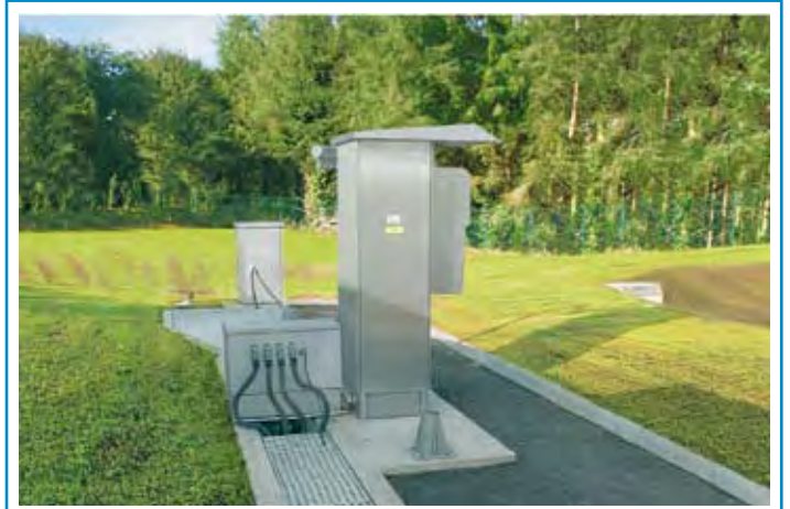
WWTP, Chateaulin, France, 8 400 m 3 /day
