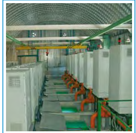
WWTP, Volgograd, Russia, 458 000 m 3 /day
