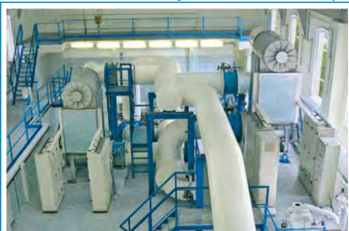
Main WTP, S. Petersburg, Russia, 864 000 m 3 /day
